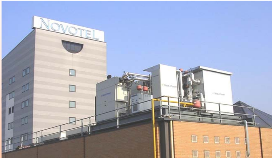
130 kW mGT trigeneration Plant
