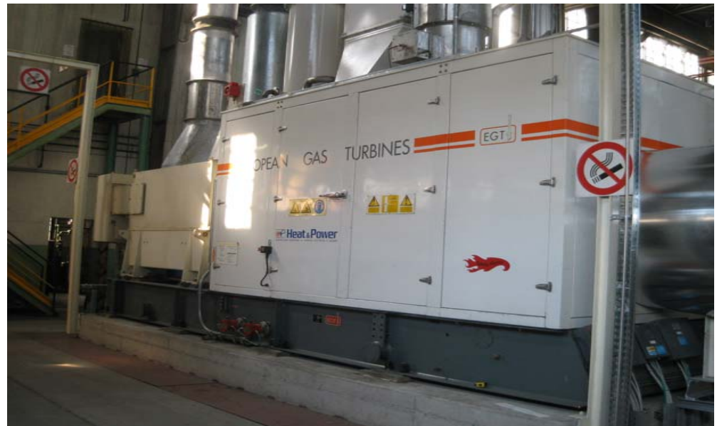
4.800 kW GT Cogeneration Plant
