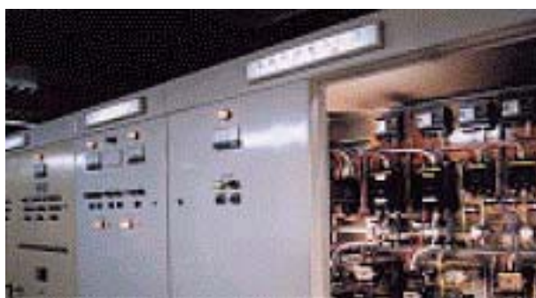
Picture 1. Installation of automatic electric power measuring instrument
