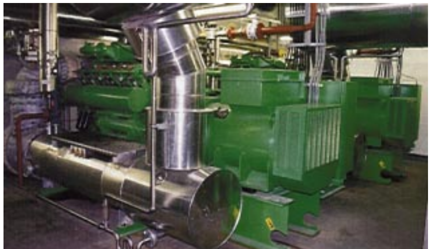
Small scale cogeneration in municipal buildings requires special attention if it is to flourish
